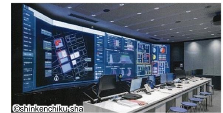
Central monitoring room for area energy management
