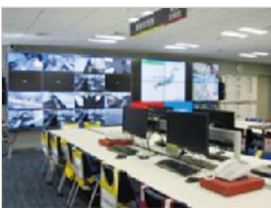
Disaster Countermeasure Headquarters (Mitsui Building No. 2)
