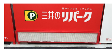
Exhaust gas panel with photocatalytic filter installed at Mitsui Repark's Enkobashi-cho No. 3 Parking Lot in Hiroshima
