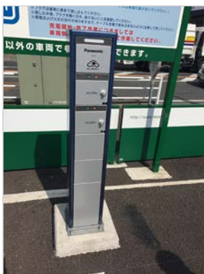
EV and PHV charging station at the Mitsui Repark Henn na Hotel Maihama Tokyo Bay Parking Lot (Urayasu City, Chiba)
