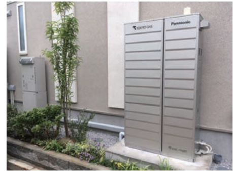
EneFarm fuel cell-equipped Fine Court residence
