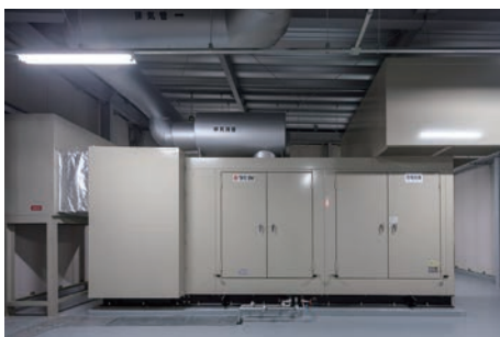
Emergency generator at MFLP Funabashi I
