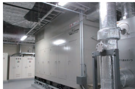
LaLaport SHONAN HIRATSUKA cogeneration system
