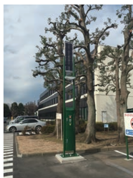
Solar LED street lighting
