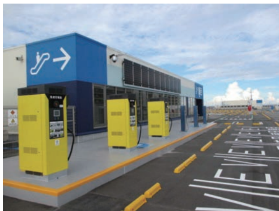
EV charging station at LaLaport SHONAN HIRATSUKA
