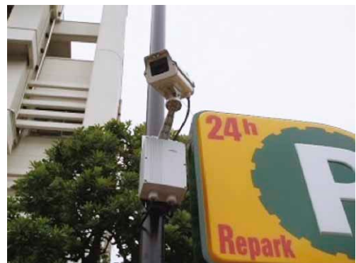
Security system installed at Mitsui Repark
