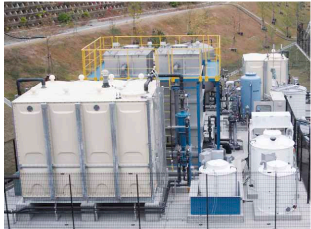
Well water purification equipment (EXPOCITY)
