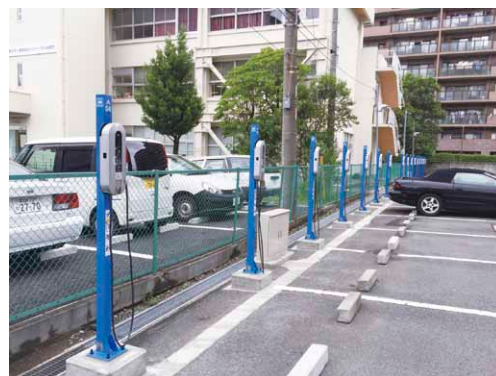
Electric vehicle and plug-in hybrid vehicle recharging stations installed with NEC Corporation (Mitsui Repark Minamiyawata 5-Chome No.3 Parking Lot: Recharging stations for 20 vehicles)
