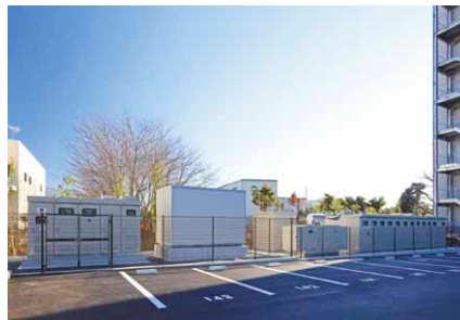
Emergency power generators (MFLP Kashiwa)
