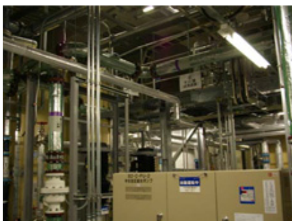
Emergency water well and filtration equipment
