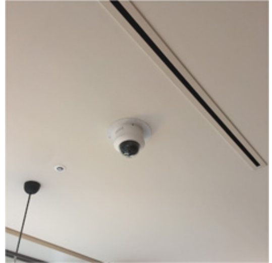
A surveillance camera installed in the Kasumigaseki Building
