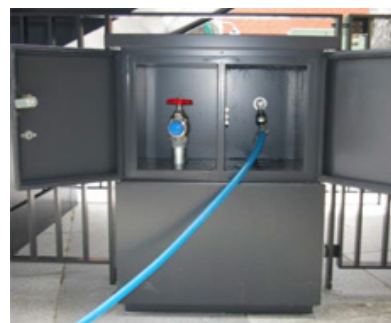
Water supply tap
