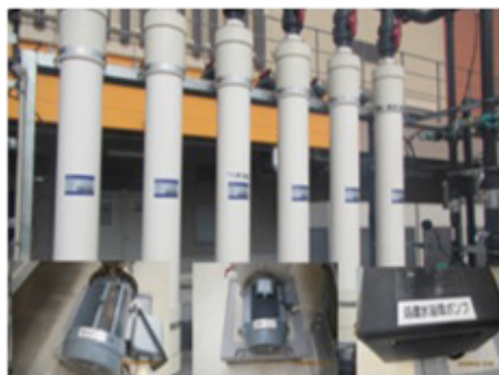
Emergency well at LaLaport Izumi
