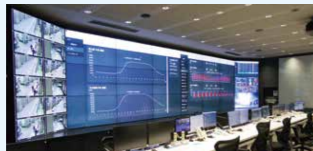
Central Control Room (Nihonbashi)
