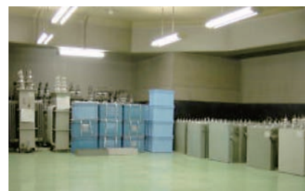
PCB廃棄物の適正保管
